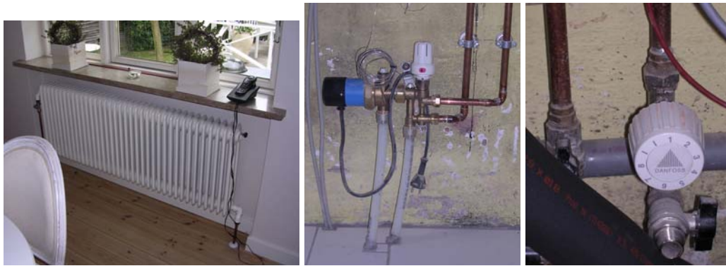
Fig. 15 Cast iron radiator in the dining room (left), the pump with integrated mixing valve for the bedroom in the basement (middle) and the return flow control thermostat valve for the floor heating in the bathroom in the basement (right).
