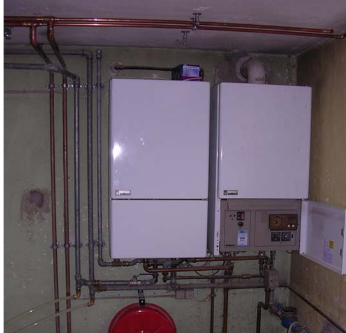
Fig. 19 The non condensing natural gas boiler (right) and the hot water tank (left).
