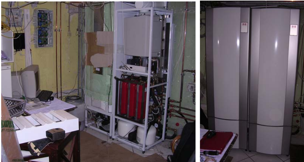
Fig. 25 Installation after set in operation on 22/6-2006 (left) and after closing the cabinets with the cover plates (right).
