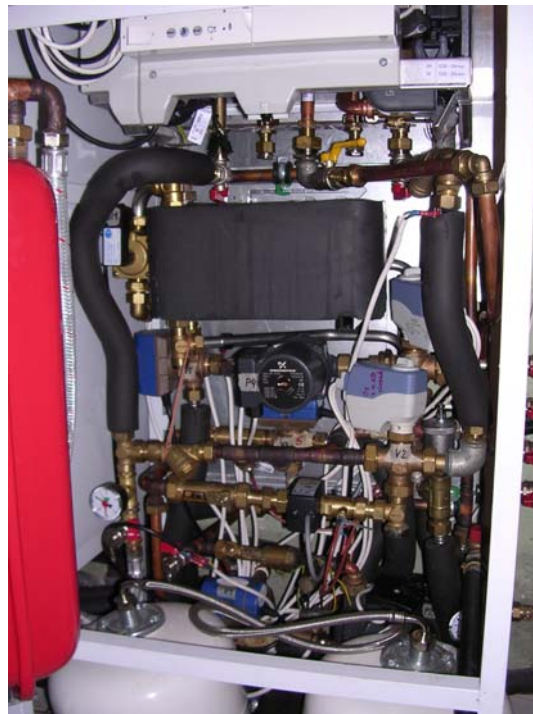
Fig. 24 Hydraulic unit inside the technical cabinet in the demonstration system; the big black box is the insulated domestic hot water heat exchanger, below the main pump P4 can be seen.
