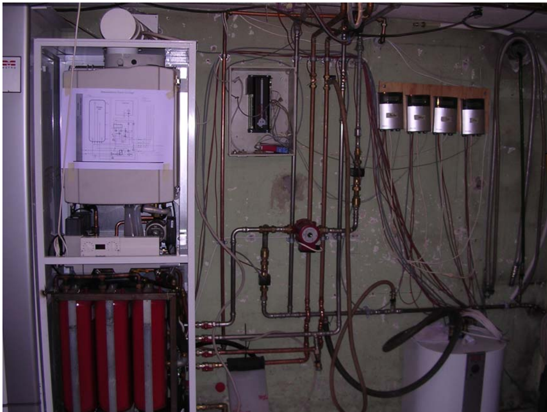
Figure 34 Measurement equipment for the new solar combisystem; in the grey box the datalogger DT500; on the right, four of the energy meter are mounted on the wall.
