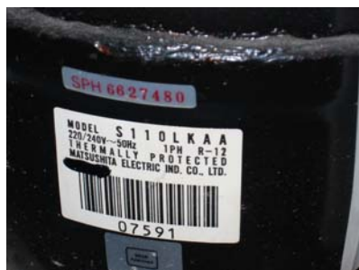
Figure 4 Plate on a compressor at the back of a refrigerator, showing the type of refrigerant used in the system. Note the text R-12.
