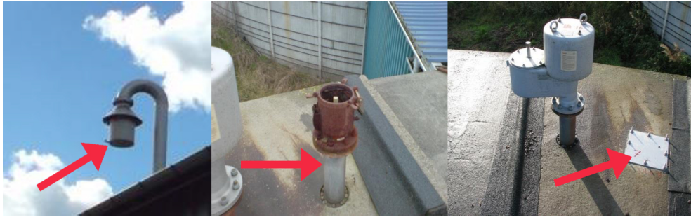
Figure 18: Examples of valves on biogas plants. The picture in the middle is an old valve not in function and leaking methane. On the picture to the right it's removed and the hole closed with a metal plat. (Stefanek, Hansen, & Rasmussen, 2015).
