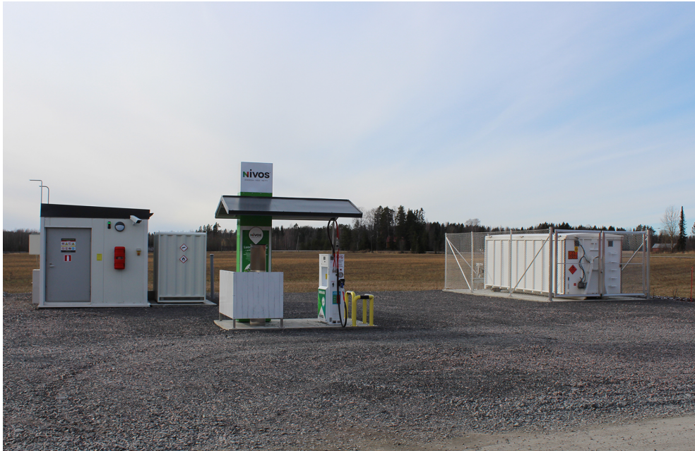
Figure 20: Example of farm scale fueling station and gas storage container in Palopuro, Finland.
