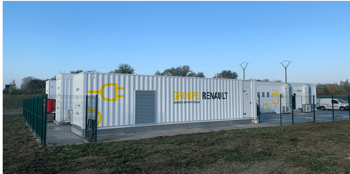
Figure 11: Batteries from Renault EVs are reused for stationary purposes 36
