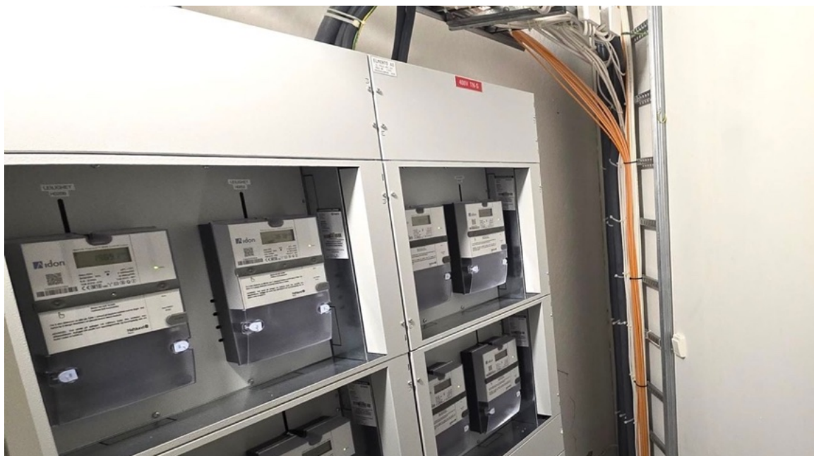
Picture: Electrical equipment at pilot site, Norway 2026
